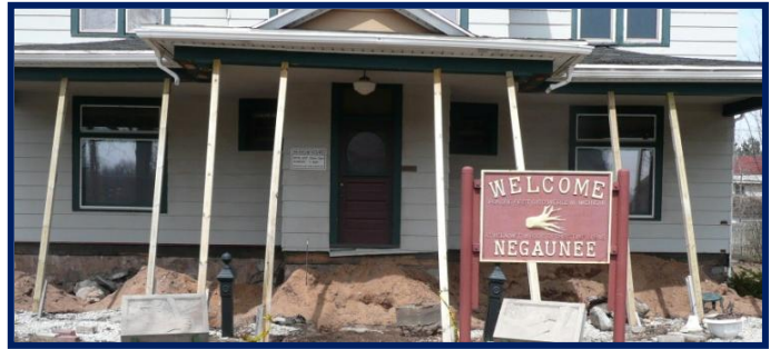
Porch roof being held up by posts– November 2011
